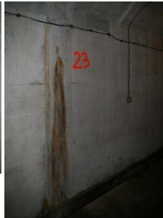
Fig. 2. Water leaking through gallery wall.
